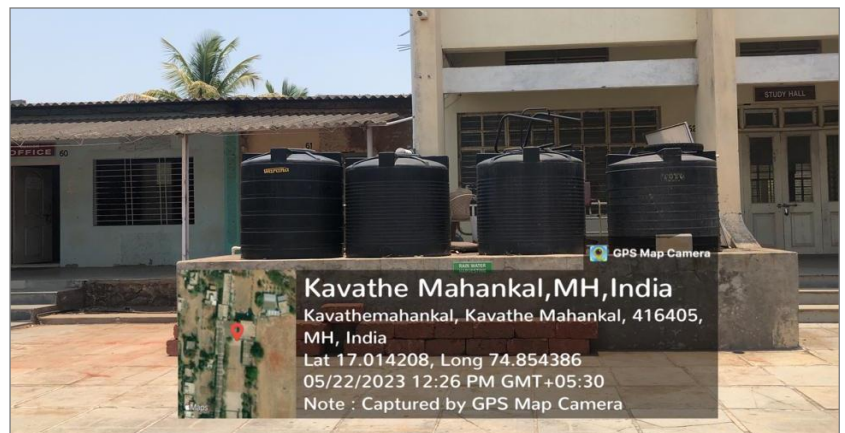
Rain water harvesting facility in the premises
